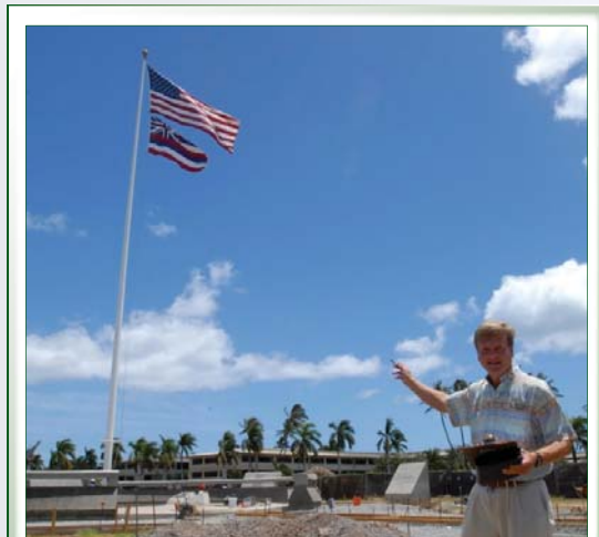
Mr. O'Donnell oversees construction of the World War II "Atterbury Circle Memorial of Heroes."
