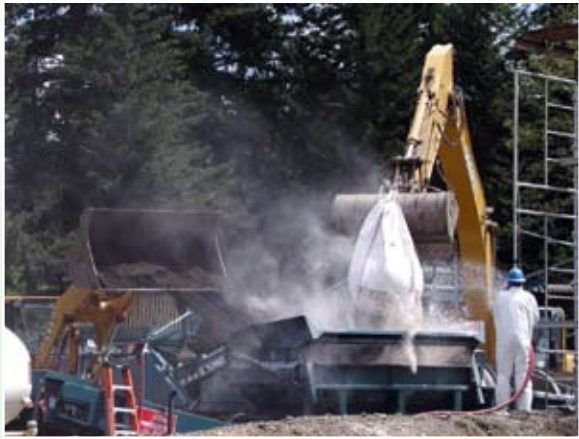
At the former Evergreen Infiltration Range, a phosphate-based stabilizer is added to prevent lead in the soil from leaching during a soil recycling project.
