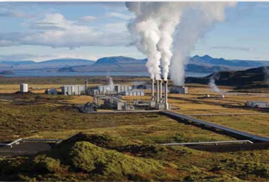
..... Steam rising from the Nesjavellir Geothermal Power Station in Iceland. Photo credit: Gretar Ívarsson
