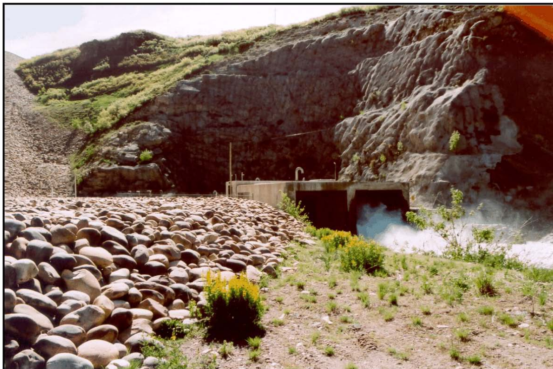
Figure 2. View of the proposed hydroelectric power plant construction site; view to the north-northeast.
