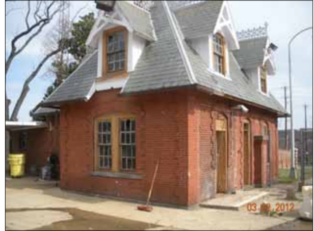
The old St. Elizabeths gatehouse is being rehabilitated on the West Campus. (photo courtesy GSA)
