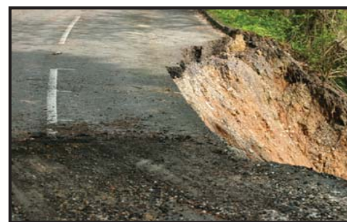
Road damage created by landslide
