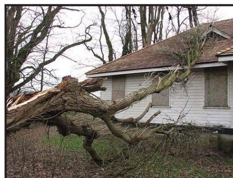
Hurricane wind damage
