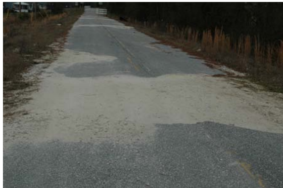
Road damage from sinkhole / soil instability
