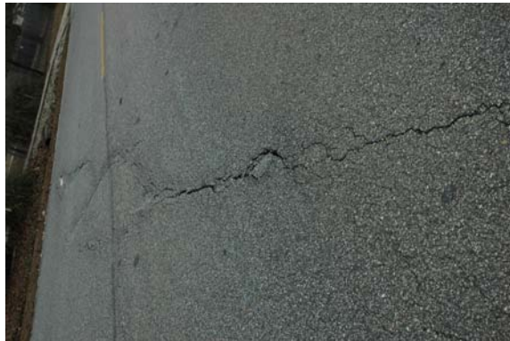
Road damage to sinkholes / soil instability
