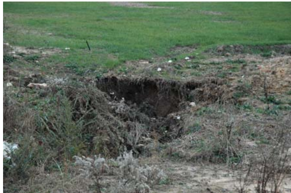
Sinkhole off of Lee County Rd#166
