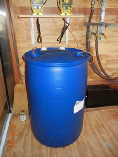
Substrate & Metering Pumps
