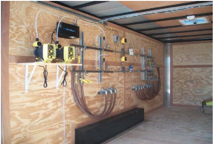
Manifolds & Metering Pumps
