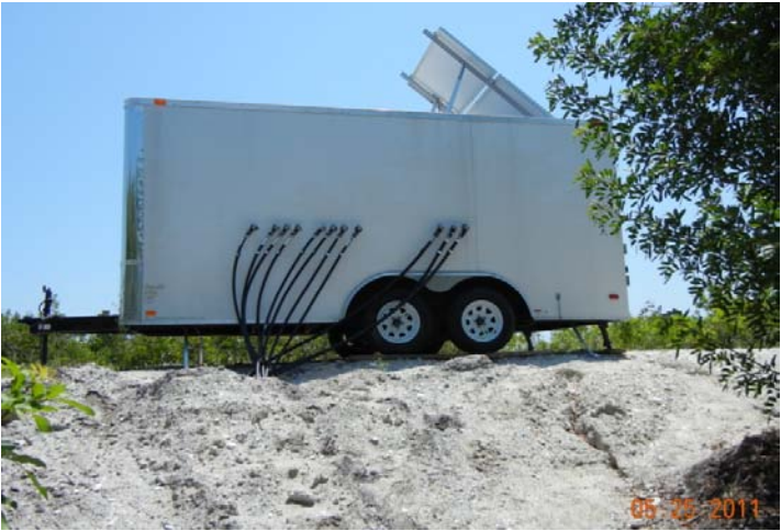
System Stub-outs (view from West)
