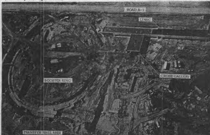
Aerial view of the NAL accelerator system "injection area." The Cross Gallery work extends downward from the Linac. Excavation for the Transfer Hall is at the bottom. The photo provides dramatic evidence of the progress in construction work at NAL since its initial groundbreaking last December 1. This photo is looking westwards; the Fox River and Batavia are less than a mile to the west. (Photo by Don Mendenhall, NAL)
