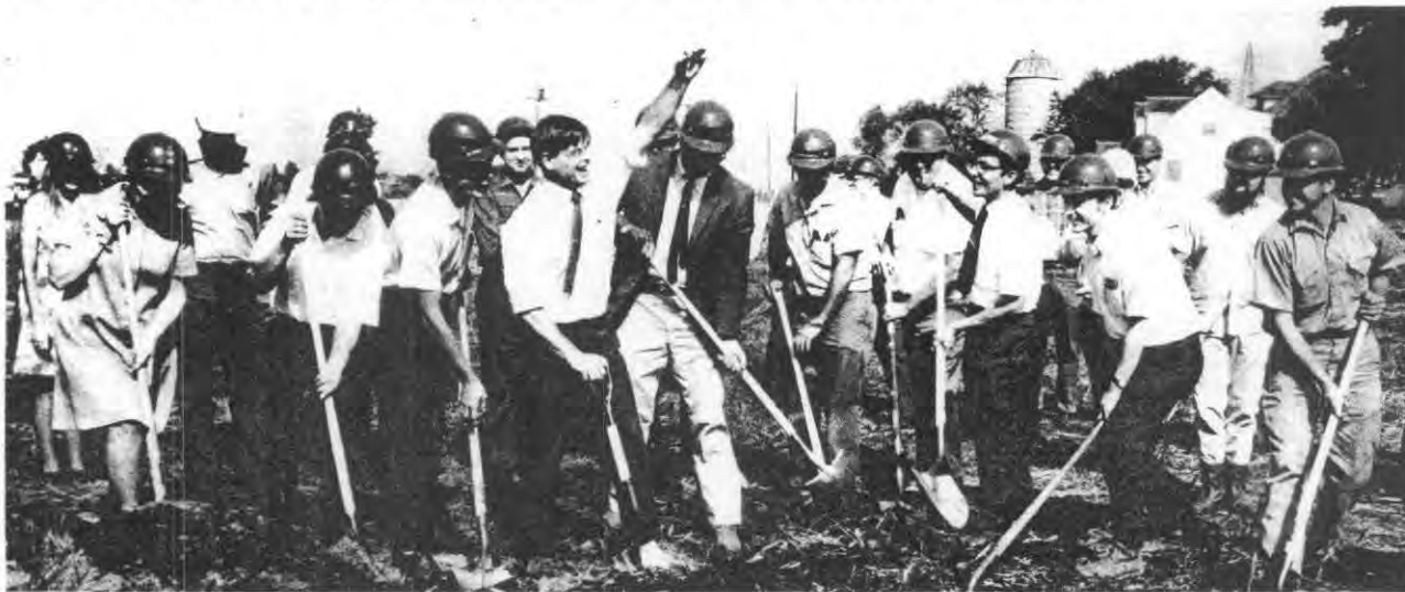
Main Ring 'ground-breaking' crews laugh as RRW exhibits ground worm he discovered in his diggings.
