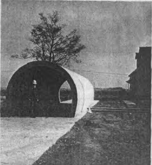
Vernon Kenney, AEC engineer, stands in front of one of the Main Ring pre-cast tunnel sections that are being fabricated at a former farm on Eola Road on the NAL site. (Photo by Tony Frelø, NAL).
