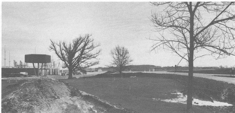
Road A and B intersection is now open to traffic. During a short ten-week period, major road reconfiguration and shielding improvements were completed.
