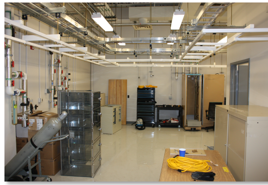
Cryogenic materials & electronics measurement lab
