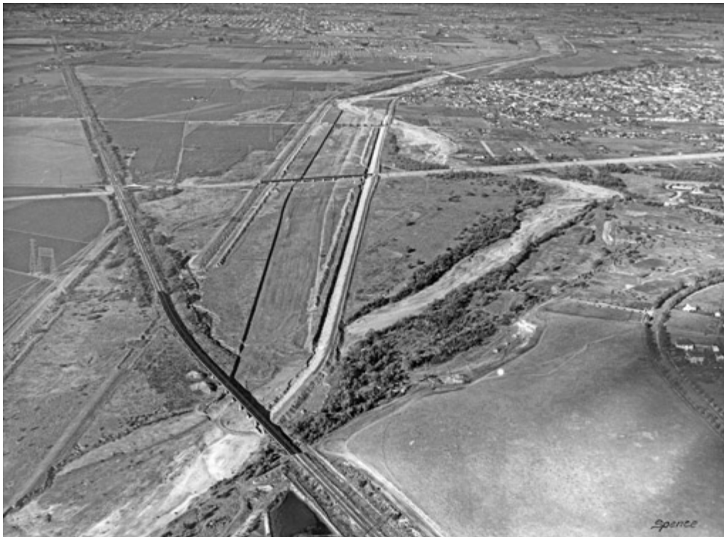
FIGURE 2.5. Levees being constructed along the Los Angeles River near Cerritos in 1932. Photograph E-3848 from Spence Air Photo collection.
