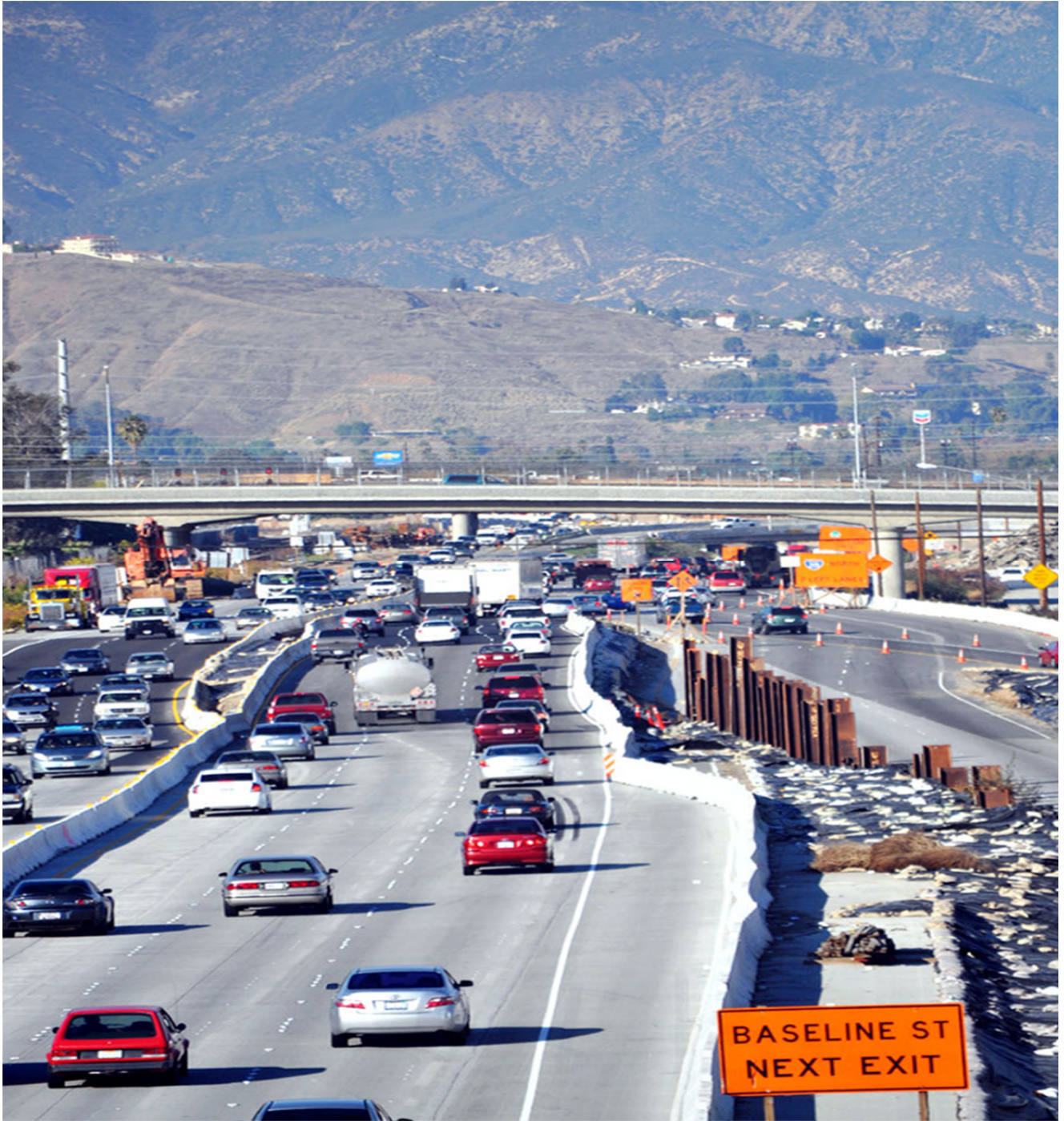
Reconstruction of the I-215 Freeway through San Bernardino spanned over seven years, from 2007-2013, at a cost of $723 million.
