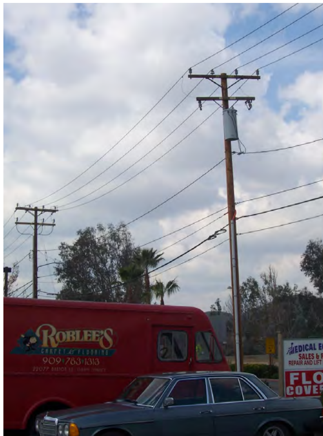
POWER POLES AND POLE-MOUNTED TRANSFORMERS ALONG BARTON ROAD
