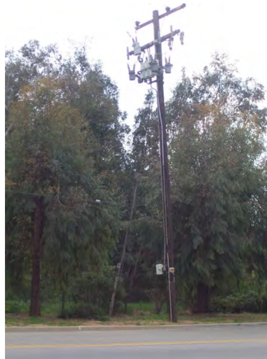
TRANSFORMER LOCATED ALONG LA CROSS AVENUE NEAR BARTON ROAD/I-215 INTERSECTION.
