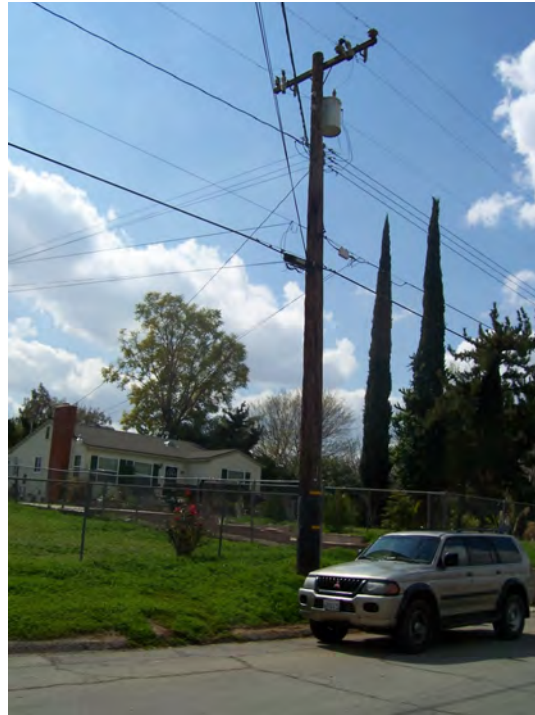
ADDITIONAL POLE-MOUNTED TRANSFORMERS LOCATED ALONG DEBERRY STREET.
