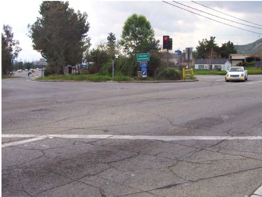
INTERSECTION OF LA CROSS AVENUE, BARTON ROAD AND THE SOUTH-BOUND 1-215 ENTRANCE, WEST OF 1-215
