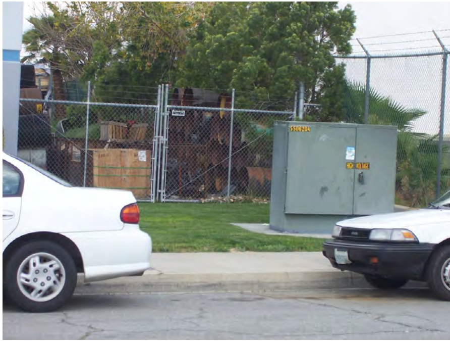
EMPTY DRUMS STORED AT COMMERCIAL PROPERTY ON COMMERCE WAY. ALSO NOTE PAD-MOUNTED TRANSFORMER.
