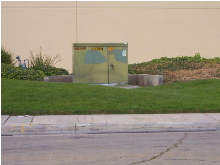
PAD-MOUNTED TRANSFORMER ON COMMERCIAL PROPERTY NEAR THE SITE.
