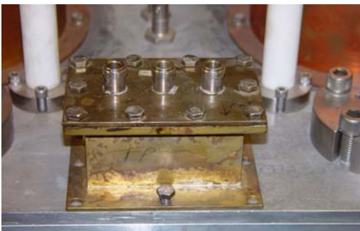
RF power splitter located on top front of the amplifier.
