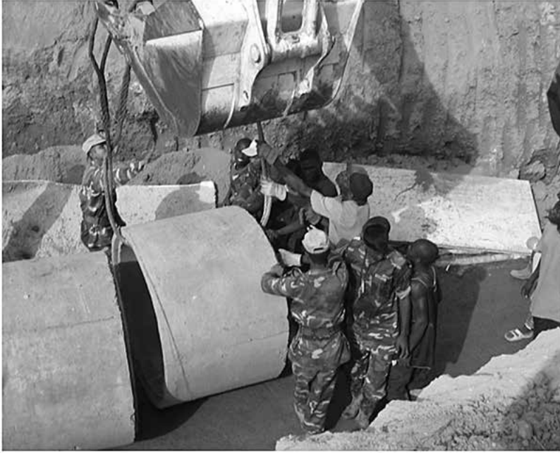
Figure 11.5. What's right with this picture? Liberian Ministry of Public Works and local personnel receive on-the-job training in culvert restoration from Bangladeshi engineers. Photo courtesy of the author.
