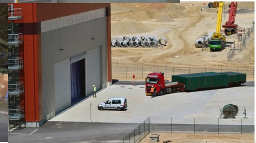
PF conductor arriving ITER site
