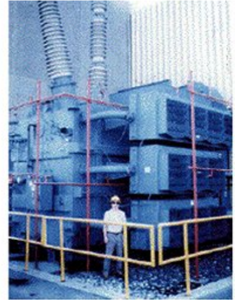
PJM Public Service Step Up Transformer
