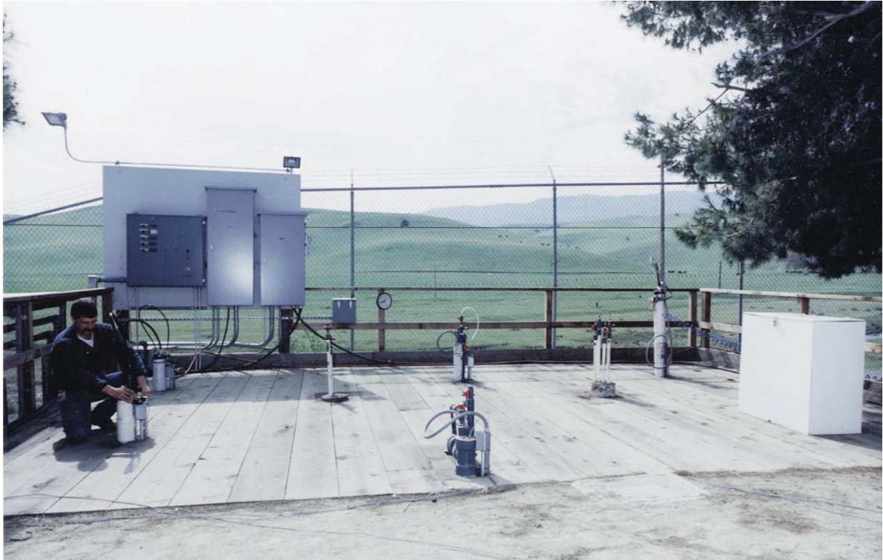
Simultaneous soil vapor and ground water extraction has effectively reduced VOC concentrations at the central GSA dry well release area.
