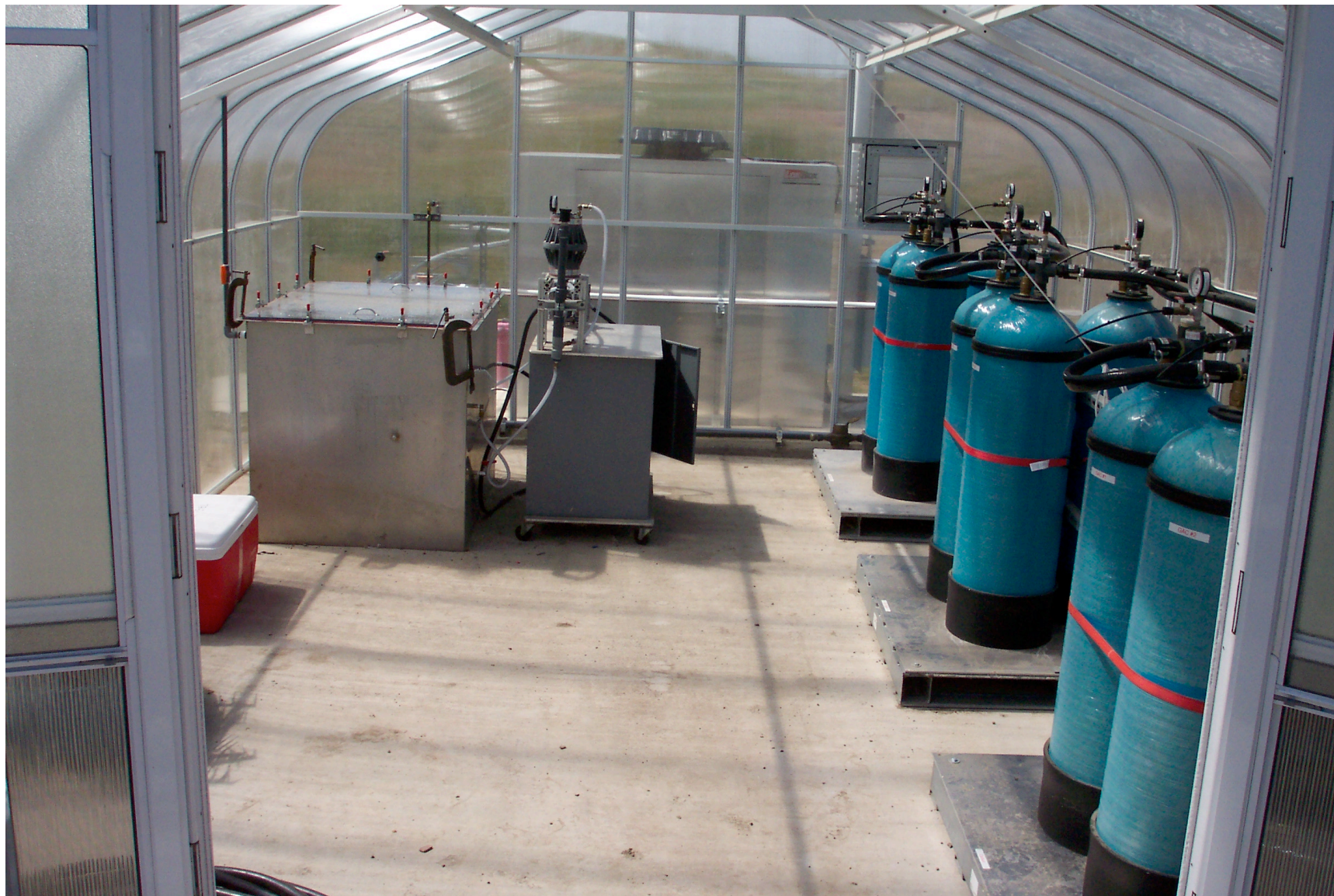
Interior of Pit 7-Source ground water treatment system showing treatment media and batch tank
