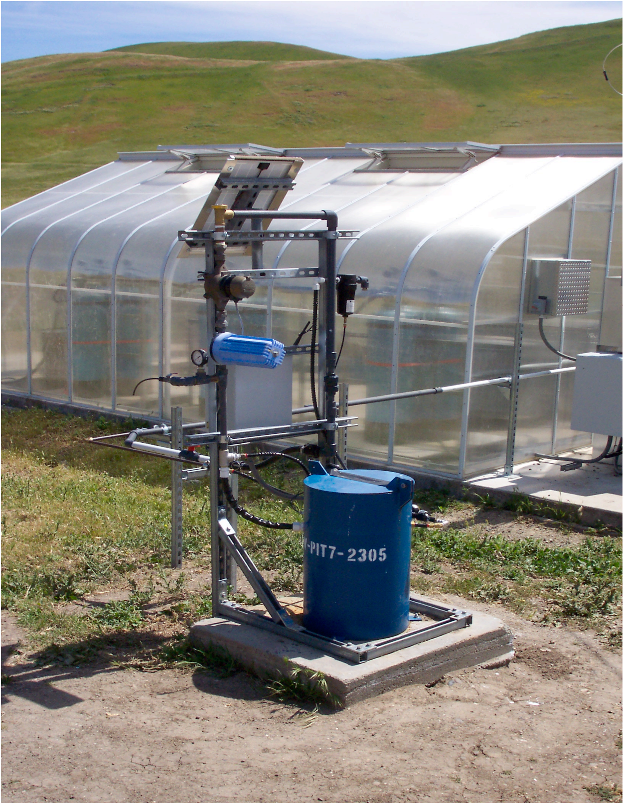
Pit 7-Source extraction wellhead manifold and solar panel
