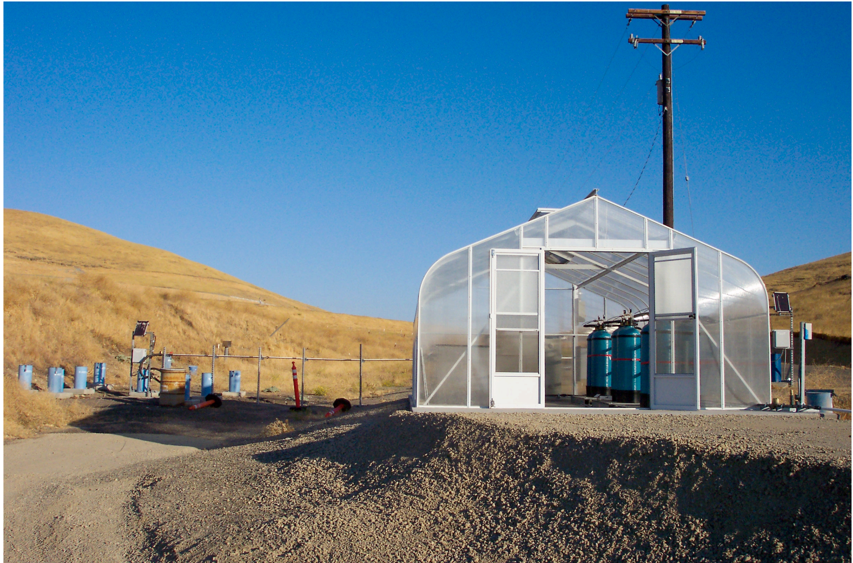
Exterior of Pit 7-Source ground water treatment system enclosure
