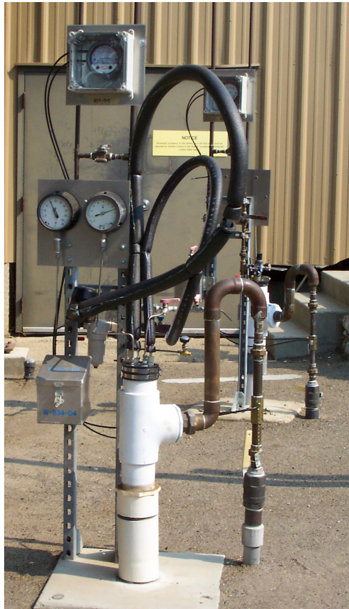
Dual-phase extraction wellhead
