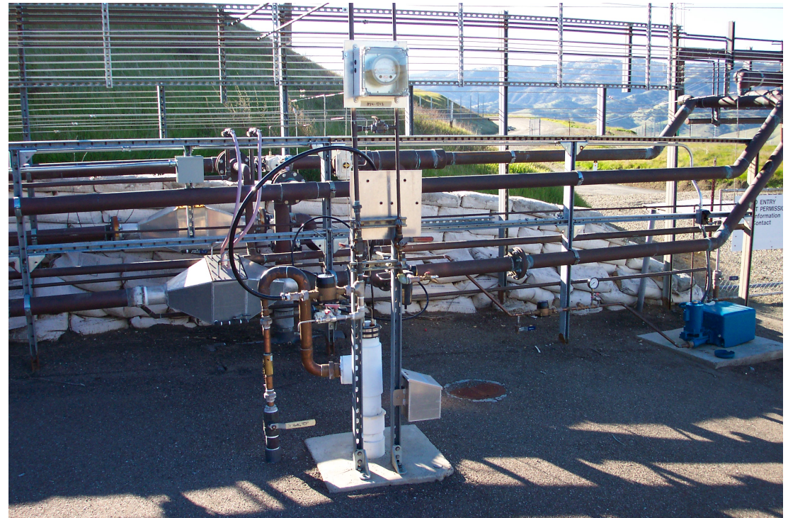
Dual-phase extraction wellhead and soil vapor and ground water pipelines.
