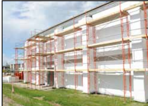
Gabriel Auditorium EIFS project is moving along nicely. Photo by Deb Ward Public Affairs
