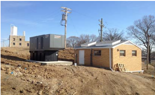
High Service Upgrade Generator
