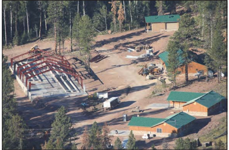
Construction of covered raceways, Administrative and residential buildings at the Ute Indian Tribe's Big Springs Fish Hatchery
