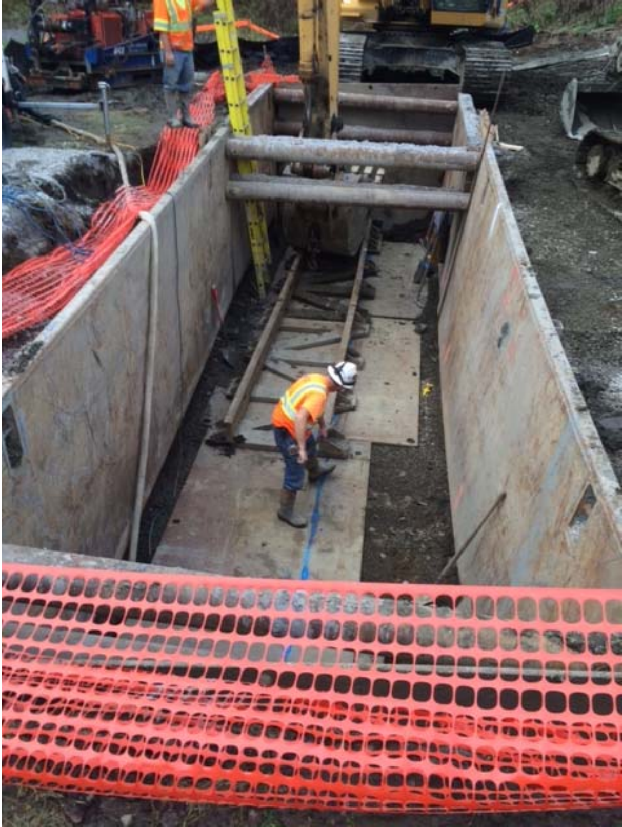
Jacking pit for the 42-inch drainage culvert that is being tunneled 8-14 feet underneath US 2.
