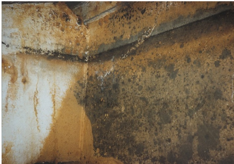
Figure 1. Stained area before wiping a small area with a rag.
