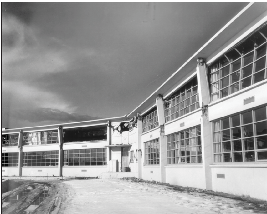
Figure 6. Earthquake shaking damage to West Anchorage High School from the 1964 great Alaska earthquake.
