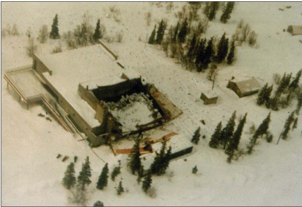
Figure 5. Aleknagik gym roof failure, snow load 1983 (photo credit John Aho).
