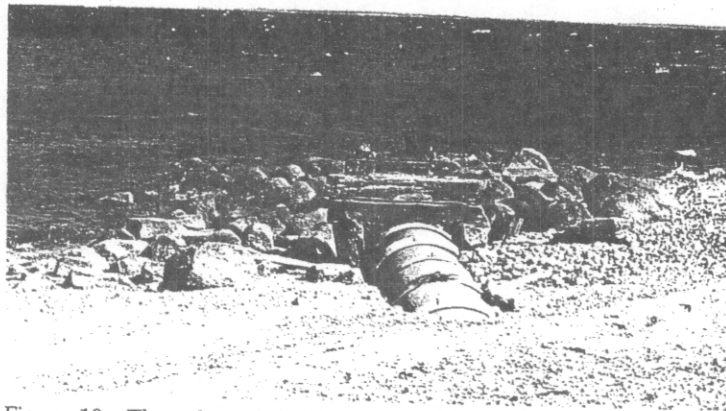
Figure 10: The culvert pipe that runs from the open channel to the bay is currently the major restriction to tidal exchange. This restriction will have to be rectified before there is much hope of the marsh becoming re vegetated with it's natural saltmarsh grasses.
