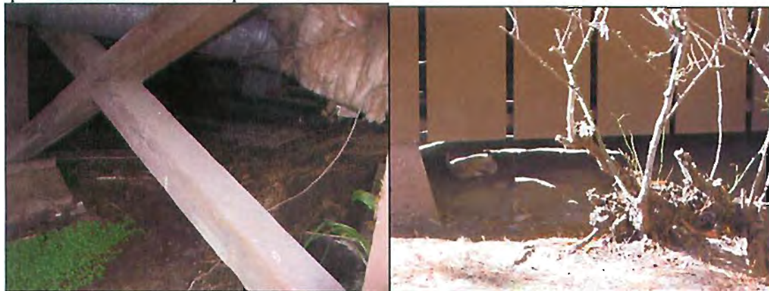
Ammonia soaked rags were placed in sub-areas to repel the raccoons, and exterior and interior of buildings were treated with Precor, an Army approved pesticide for treating fleas.
