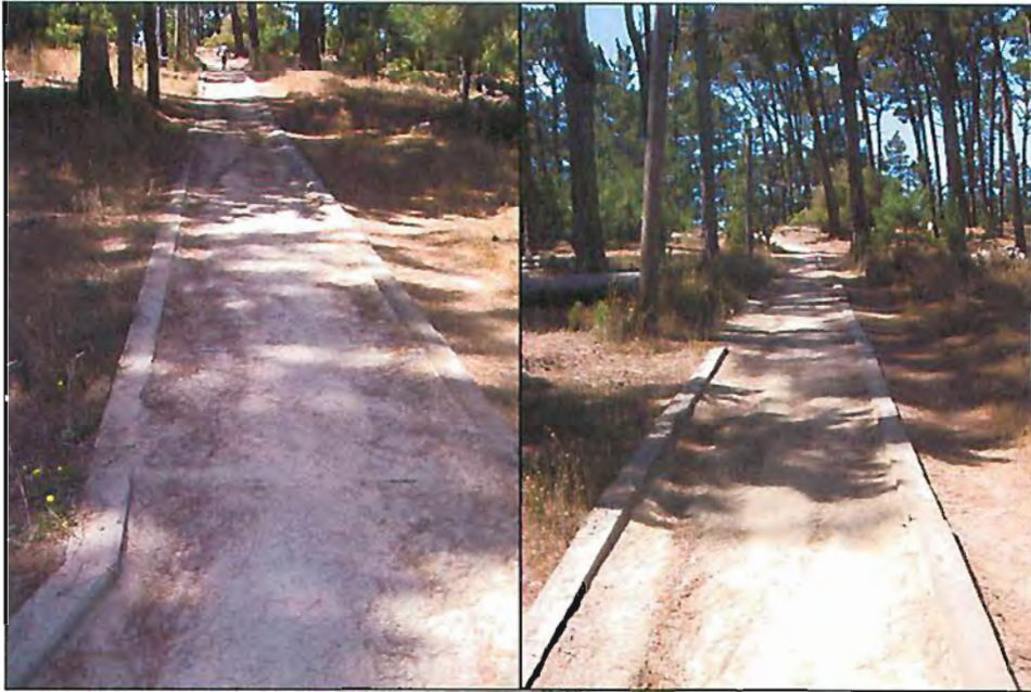
Water flows down the trail dislodging decomposed granite, and creating gullies and an uneven surface.
