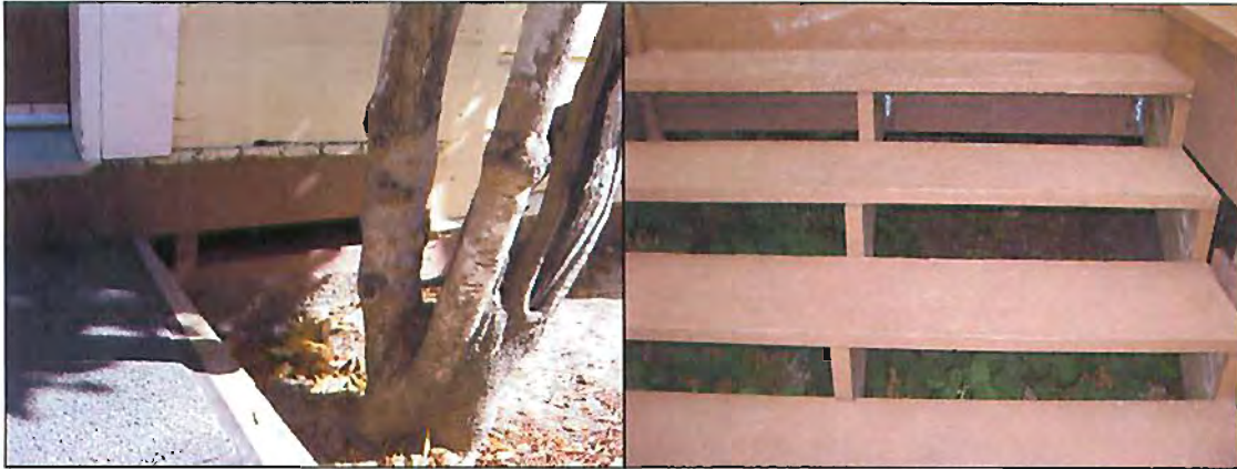
Raccoons can easily access sub-areas of the historic POM lodging buildings
