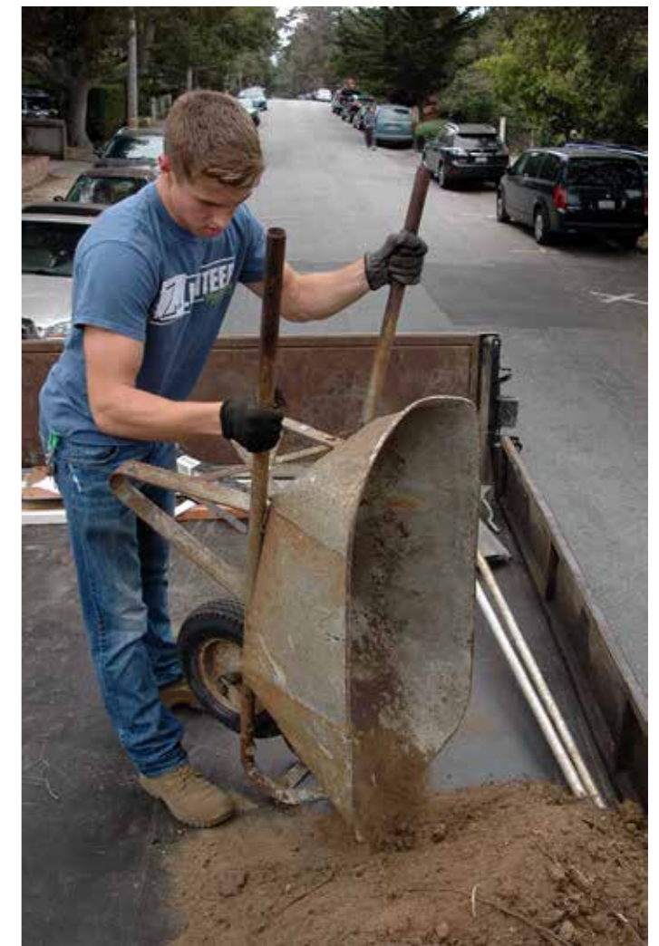
Pfc. Zachary Chapman dumps a load of dirt from the grading project Sept. 10 at the American Legion Post 512 in Carmel.
