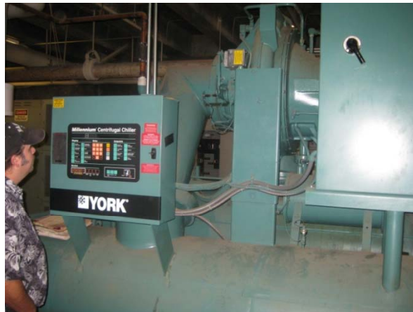
Courtesy York/Johnson Controls
