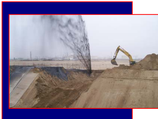
Encroachment over Pipeline
