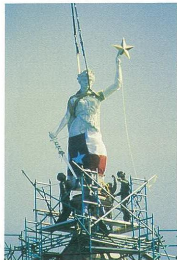
Above: CH-54A “skycrane” makes easy work of lowering the Goddess into place.
