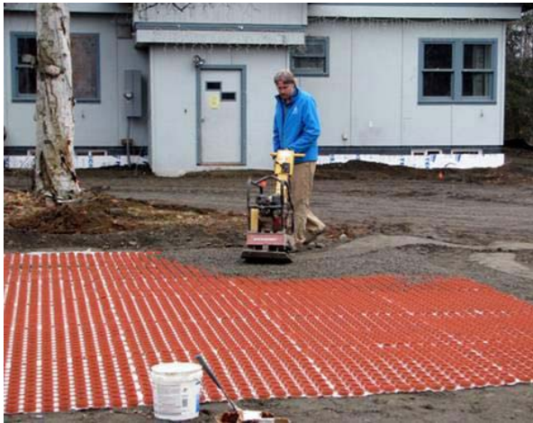
Figure 2. A Kenai Watershed Forum staff member applies the last layer of gravel on a new GravelPave2 system in front of the historic Soberg House at the confluence of Soldotna Creek and the Kenai River.
