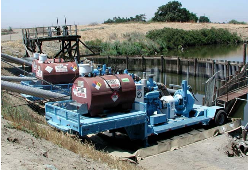
Figure 4: Example of Temporary Pump and Generator Units
