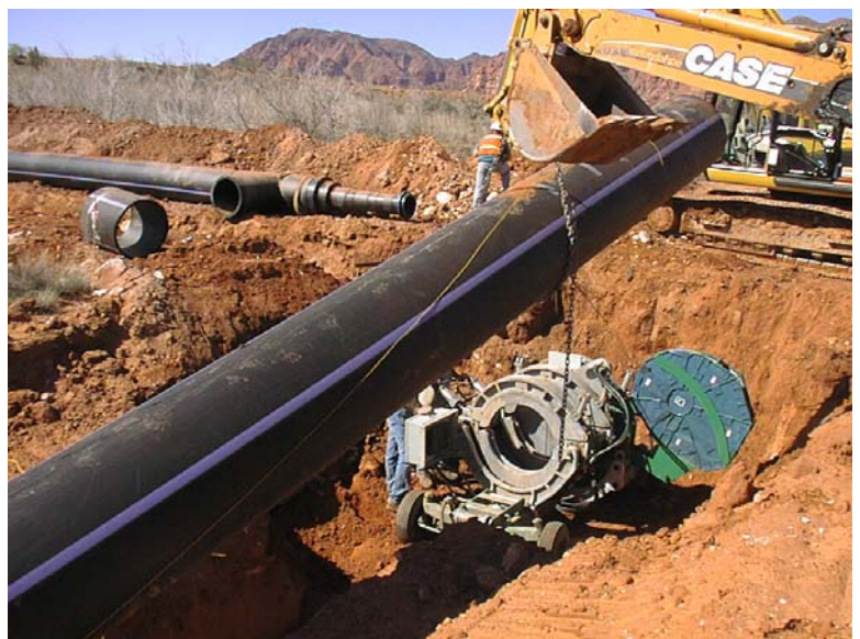
St. George has already built sections of its eight-mile pipeline to deliver reclaimed water to the Shivwits Indian Reservation. The city installed various sections of the pipe as areas along the route of the pipeline were developed. (Photo courtesy of City of St. George Water Services.)
