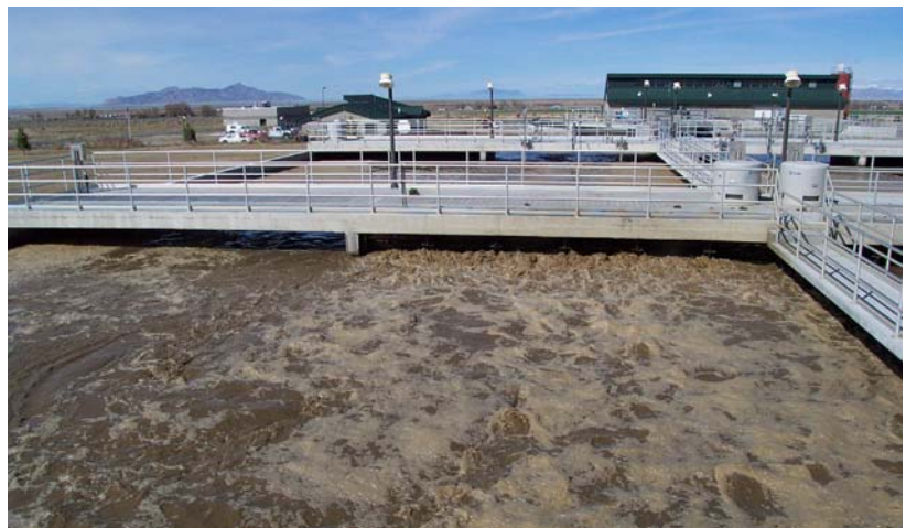
Tooele's wastewater treatment facility uses an oxidation ditch as part of its treatment process. (Photo courtesy of Tooele Wastewater Treatment Plant.)
