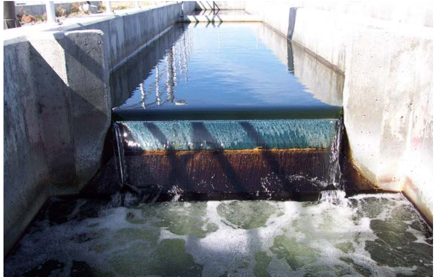
Renovated water after tertiary treatment at Tooele's Wastewater Treatment Plant. (Photo courtesy of Tooele Wastewater Treatment Plant.)
