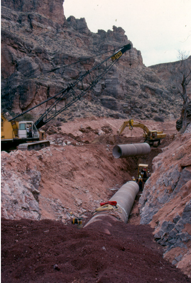
As additional water developments require long, expensive pipelines, the economics of meeting future water needs may favor a water reuse project.
