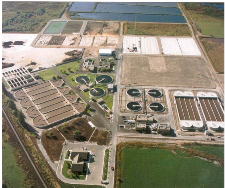
The Timpanogos Special Service District currently services several cities in north Utah County. A proposed satellite plant near Saratoga Springs will reclaim a portion of the city's wastewater for reuse while sending the removed solids on to the district's main wastewater treatment facility shown above. (Photo courtesy of Timpanogos Special Service District.)
