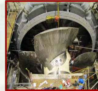
Webbers Falls Turbine
