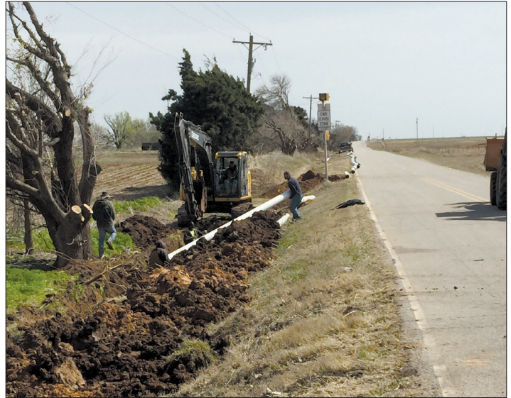
Work crew installing water main along East Willow Road to connect the Garber Municipal Authority to the Enid Municipal Authority
